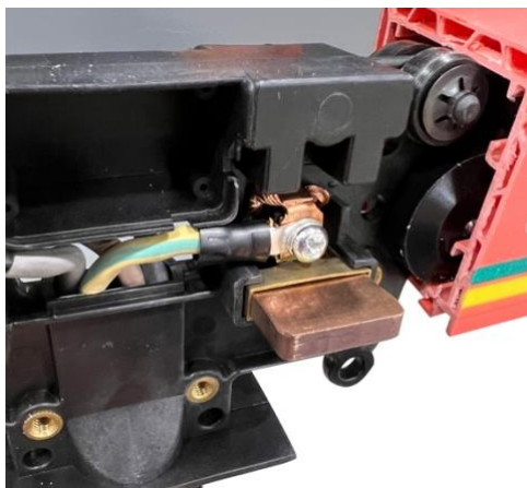
4.6.9 40 Amp Single Collector Installed
